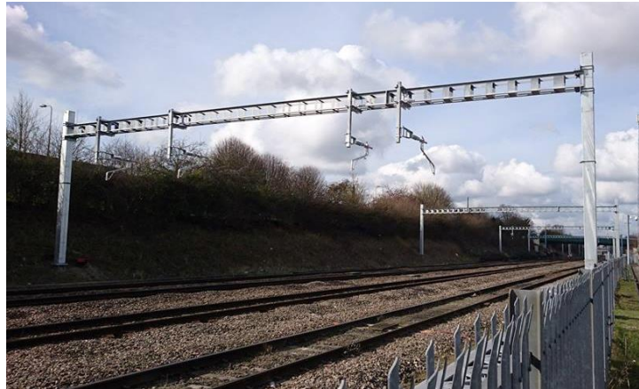
Figure 15: Electrification infrastructure near Didcot Parkway
